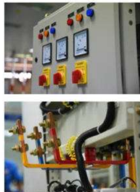
Electrical Wiring Services
